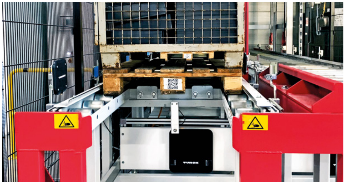
External RFID near-field antennas on the conveyor system only detect the pallet directly in front of them
